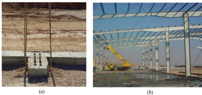
Fig. 9. (a) Accurate layout of anchor bolts using the coordinate method, (b) Assembly process of erected steel warehouse
