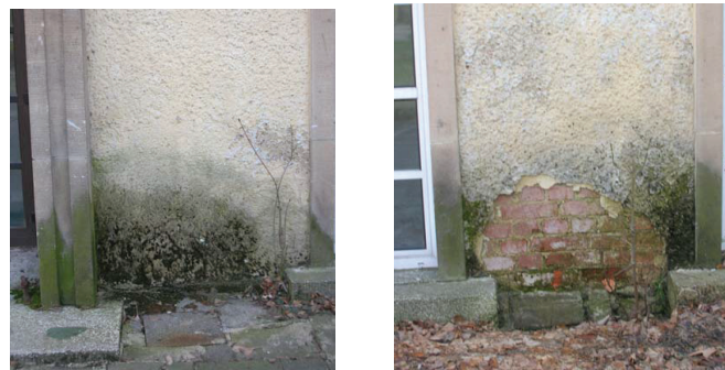
Fig. 1. Walls damaged by dampness
